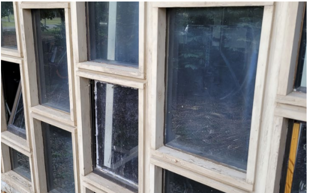
Windows at Weight Room are Particularly Weathered
