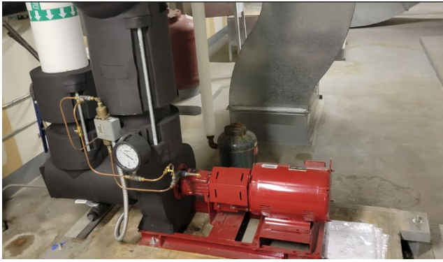
Chilled water pump
