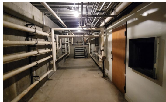
Basement Supply Air Plenum
