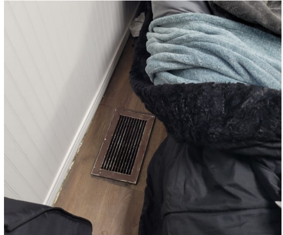
Bedroom Floor Grille
