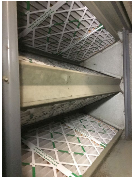
AHU-S1 Mixing box
