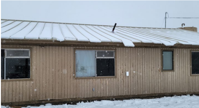
West Facing Façade Is extremely weathered. Plumbing Vent at roof has been bent by sheeting snow
