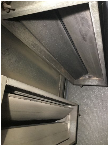
AHU-S4 Mixing Box
