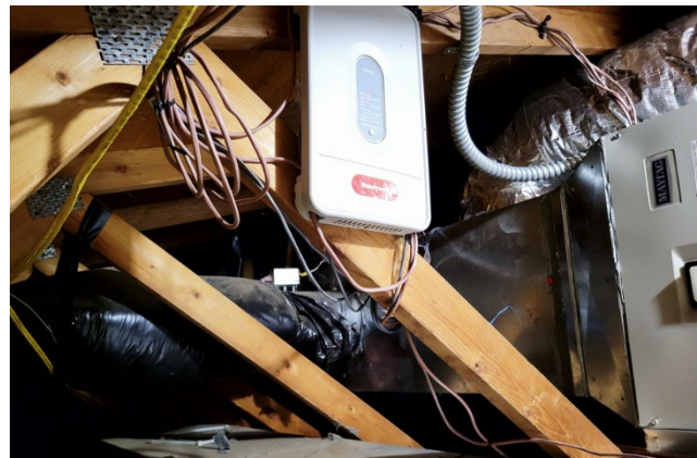
Controller for Classroom Unit
