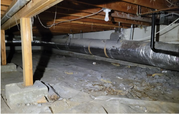
Duct Distribution in Crawlspace
