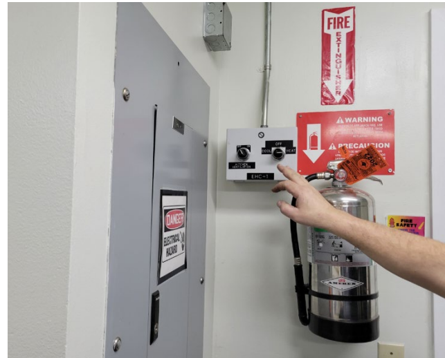
Kitchen Exhaust and Makeup Air Controller
