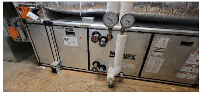
Cottage 7 AHU Cooling Coils Are Not Connected No Cooling
