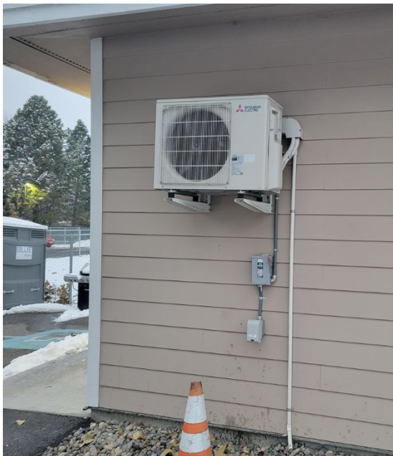
Server Room Outdoor Unit
