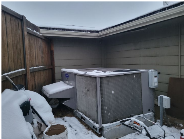
Common Area Gas Packaged AC Unit
