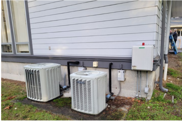
AHU-2A and AHU-2B condensing Units
