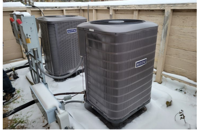
Condenser Units for Furnace
