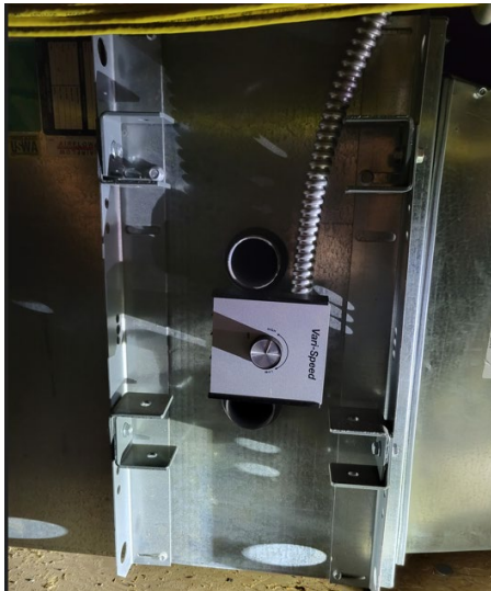
Kitchen Makeup Fan in Attic
