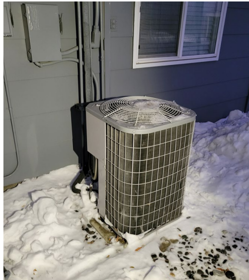
East Side Condenser Unit
