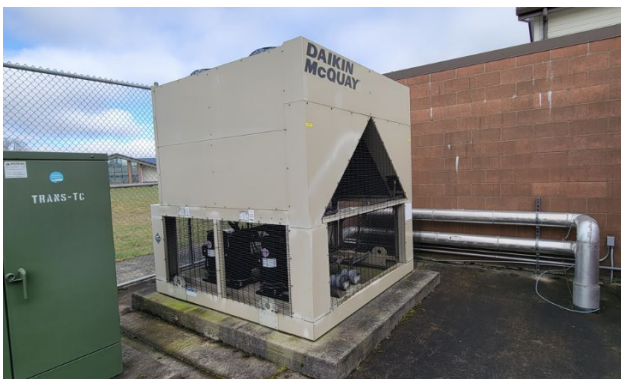
Air Cooled Chiller CH-1
