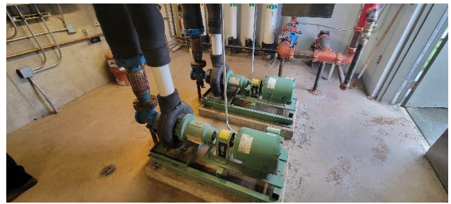
Chilled Water Pumps
