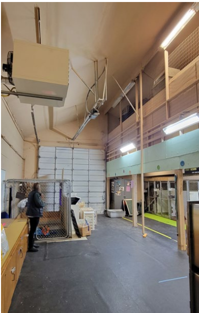
Kennel Area Unit Heater in Upper Left
