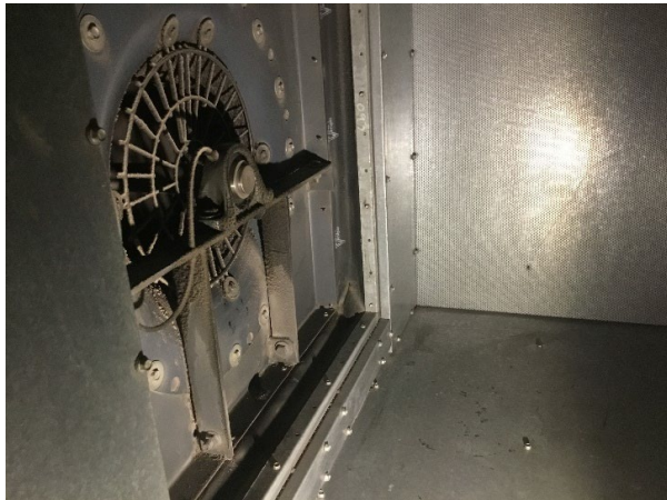
Typical AHU Return Fan Note flexible connection tear starting in lower corner
