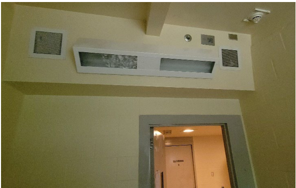
Air Grilles in Sleeping Rooms
