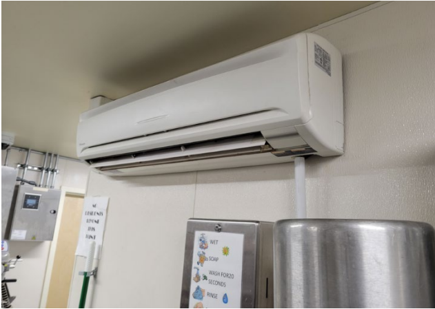
Kitchen AC Unit
