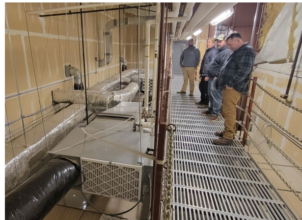
Mechanical Catwalk and HVAC Equipment above Main Hallway
