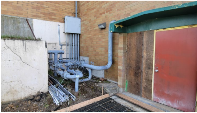
Natural Gas Service to building
