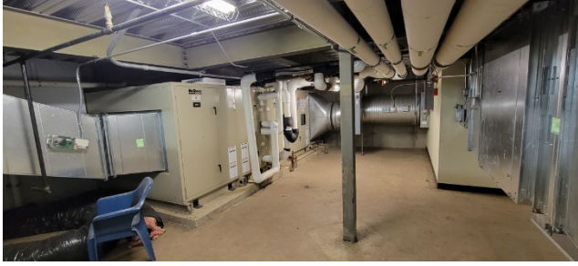
HCA Air Handling Unit (Left) & Return Fan (Right)
