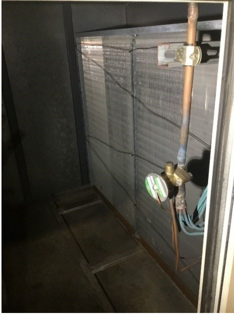
AHU-A1 Cooling Coil
