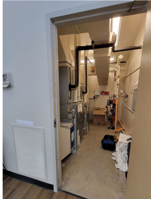
Mechanical Room for Units 2A and 2B Note common outdoor air duct to exterior
