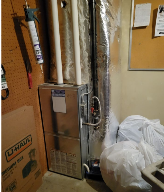
Classroom Building Furnace
