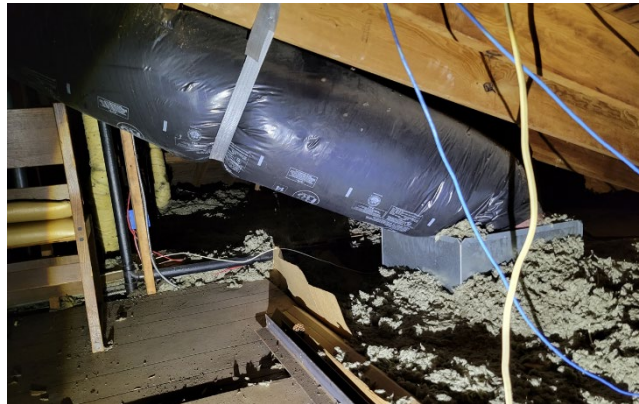
Second Floor System Return Ductwork
