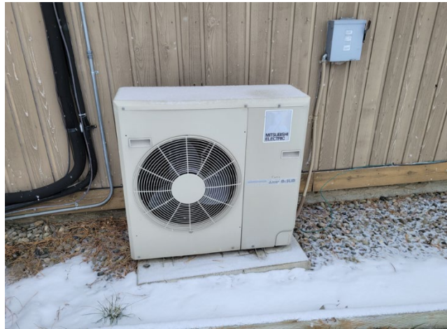
Dry Storage Outdoor Unit
