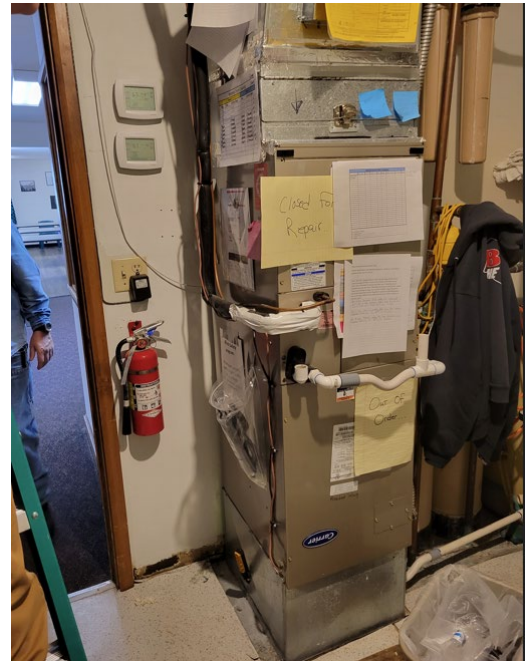
Residential Wing Furnace
