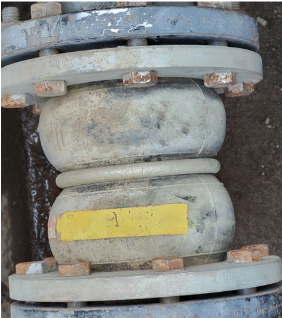
Original Expansion Coupling
