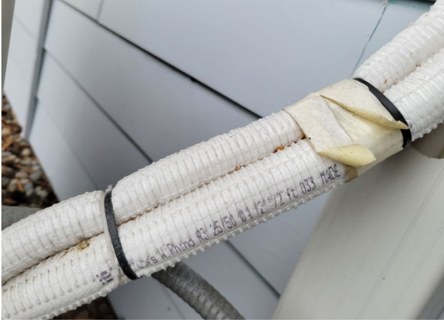
Server Room AC Unit Refrigerant Lines Appear well protected
