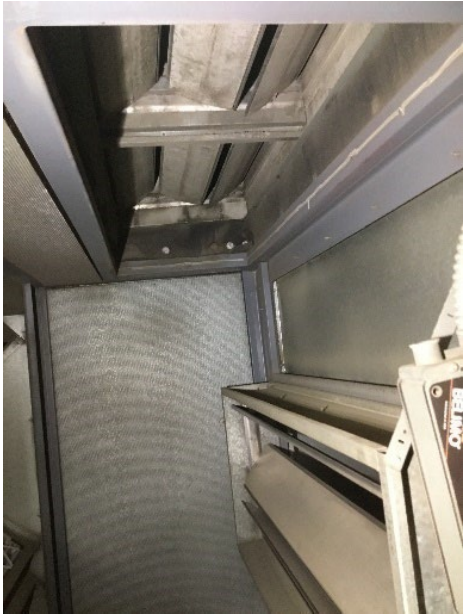
AHU-A1 Mixing Dampers
