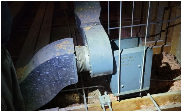
Exhaust Fans in Attic
