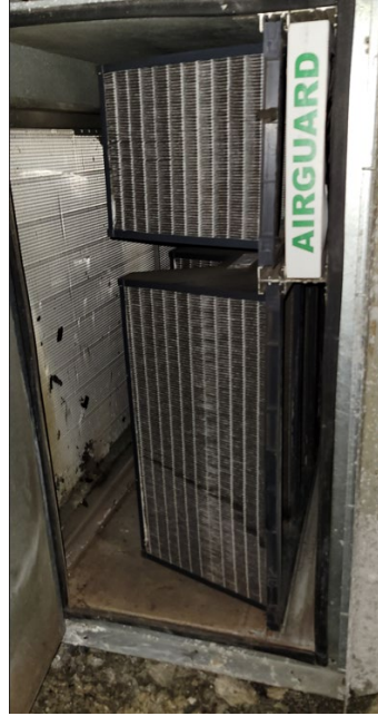
Prefilters and V-Bank Filters. Some prefilters are missing and coil needs cleaning
