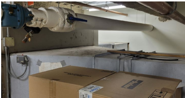
Supply ducts from AHU to basement supply plenum
