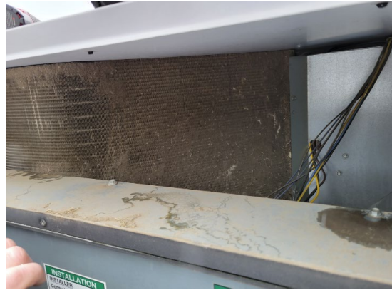
Condenser Coils Are Loaded with Dirt and Need Cleaning
