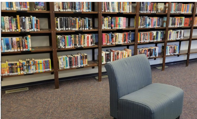
Floor Grilles Around Room Perimeter
