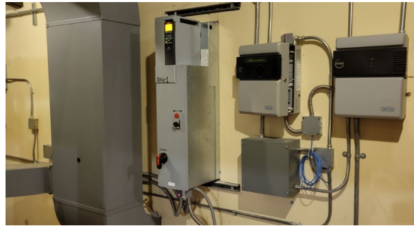
AHU Speed Drive and Control Panels
