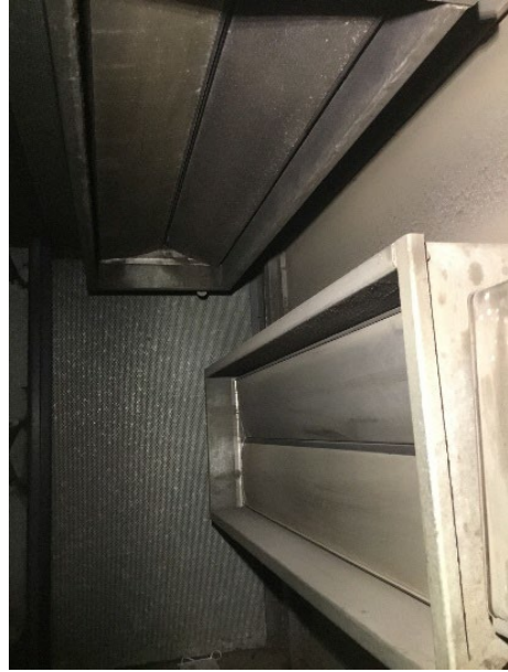
AHU-S3 Mixing Box Note: Both return and outdoor air dampers are fully closed.
