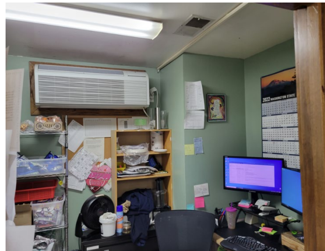
Kitchen Office with Through-wall Packaged AC
