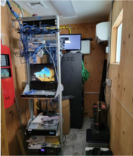
Server Room with AC Unit
