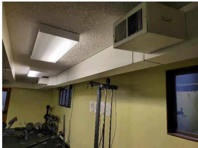
Basement Ducts and Registers in Fitness Room
