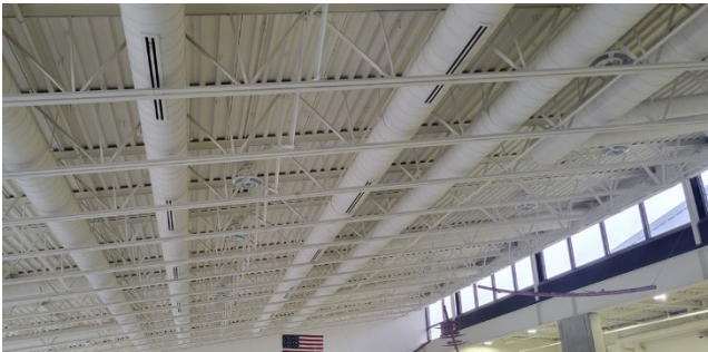
Dining air distribution with slot diffusers
