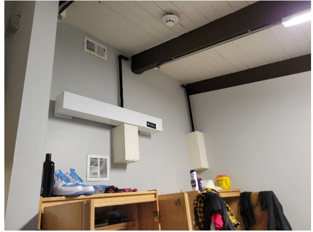
Ventilation for Typical Bedroom
