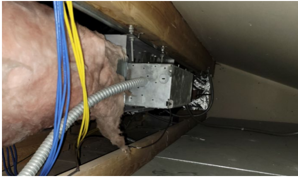
Kitchen Makeup Air Fan Coil in attic with Electric Heat
