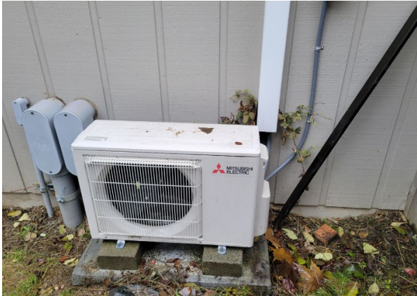
Pantry Condensing Unit
