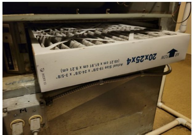
AHU-2A Filter Section
