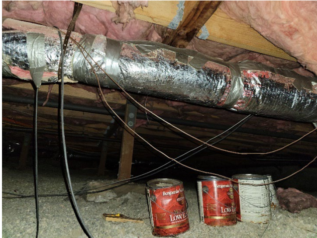
Crawspace Air Distribution
