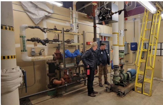
Ground level Mech room with Hydronic Pumps
