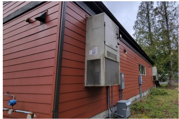
Air Conditioning Units on the Back Wall
