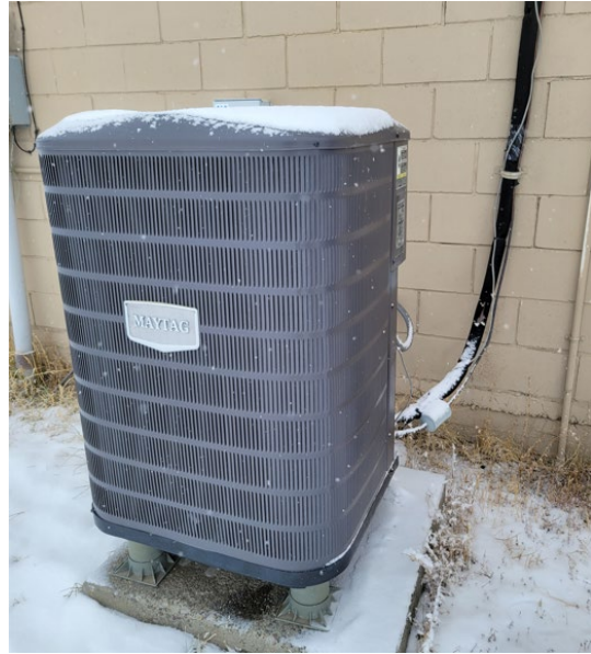
Classroom Condensing Unit
