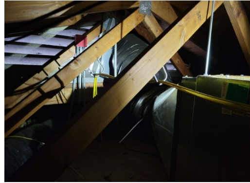
Kitchen Makeup Air Intake in Attic
