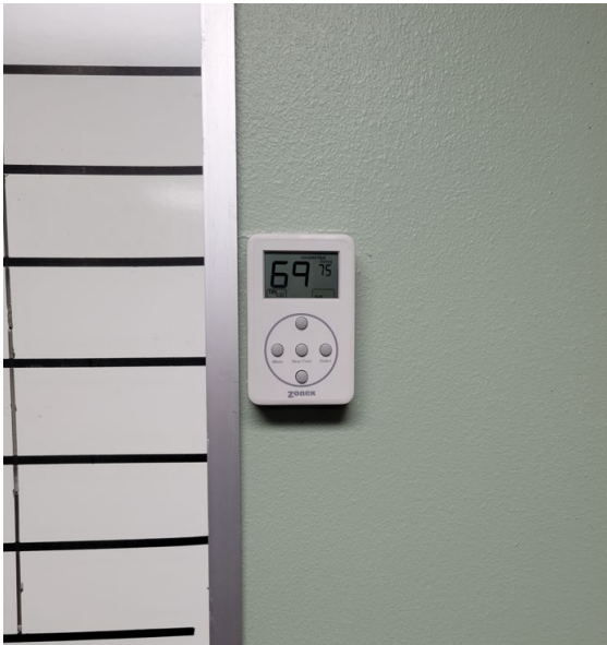
Zone Thermostat in Office
