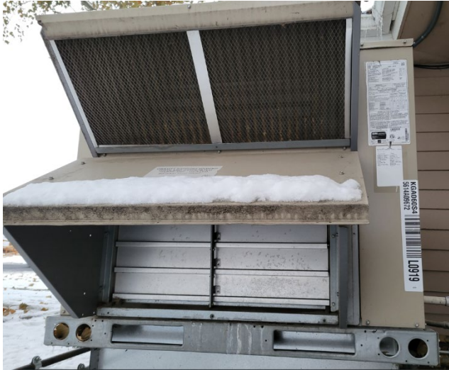
Air Handler Intake and Relief
