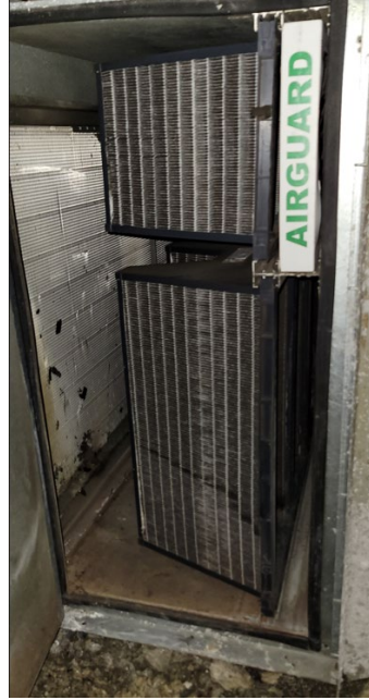
Prefilters and V-Bank Filters. Some prefilters are missing and coil needs cleaning.
