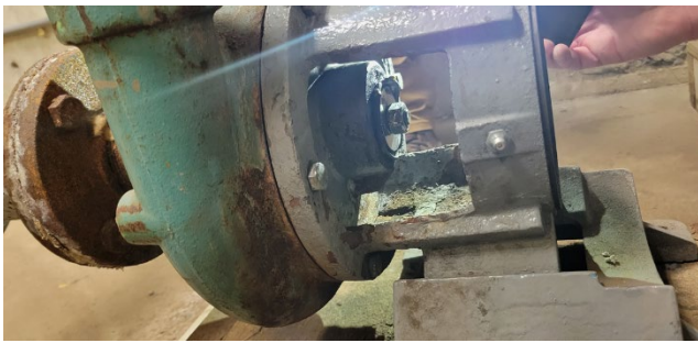
Internal pump (left above) components (motor and impeller) have been removed. This pump casing is functioning as a pipe for campus water to flow through.
