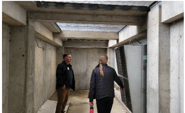
Air Intake in Area Well
