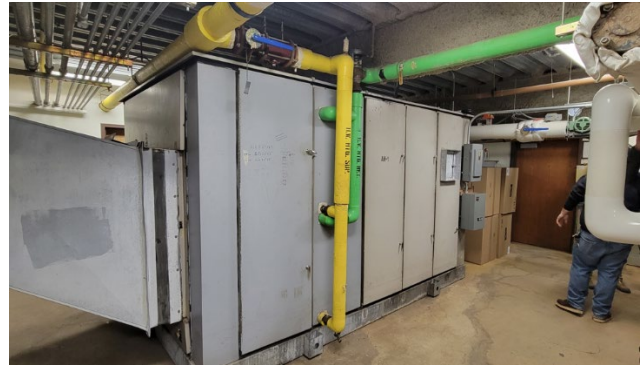
Air Handling Unit in Basement Mechanical Room
