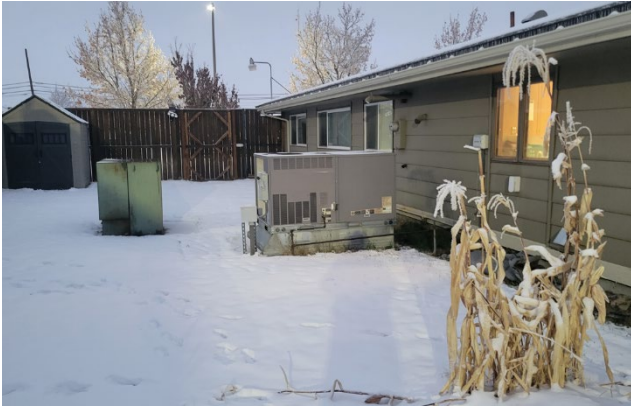
Gas Fired Packaged AC Unit Serving Bedroom Wing
