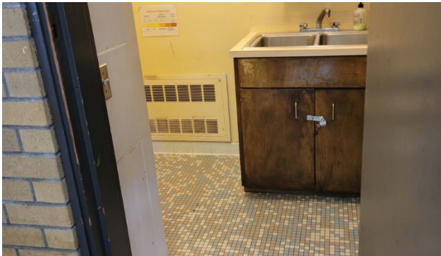
Bathroom with Heating Convactor
