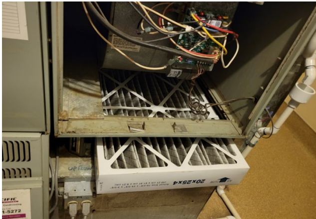
AHU-2A Filter Section
