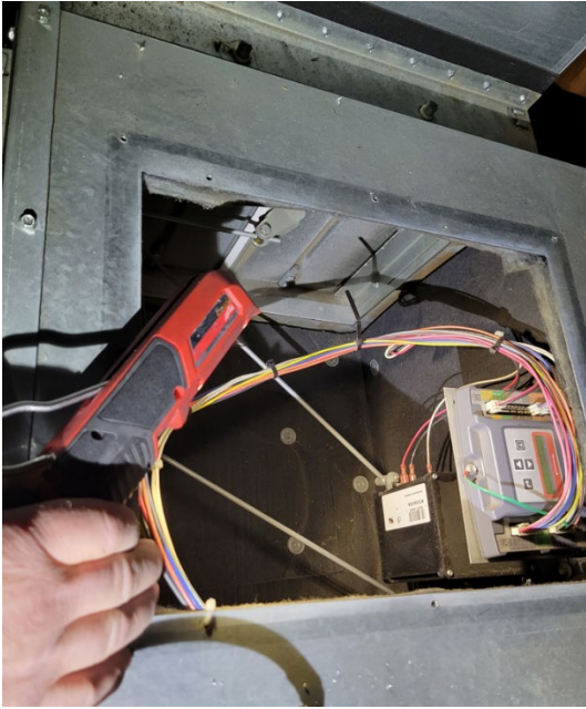
Second Floor Air Handling Unit
