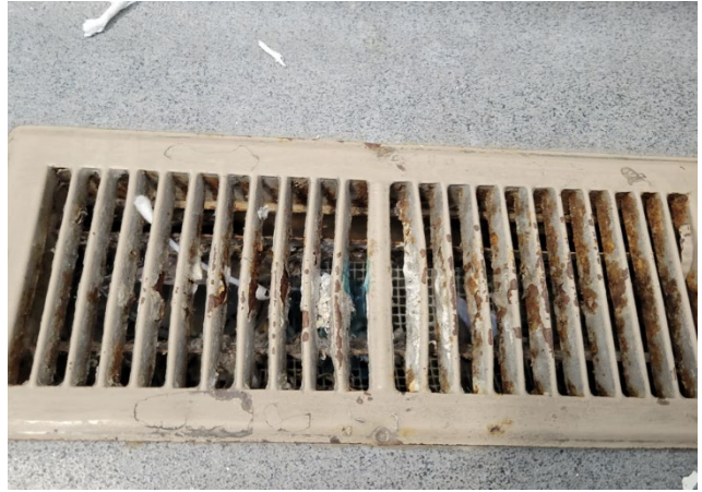
Restroom Floor Register
