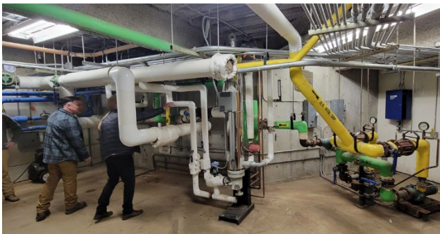
Heating and Domestic Hot Water Piping in Basement Mechanical Room.
