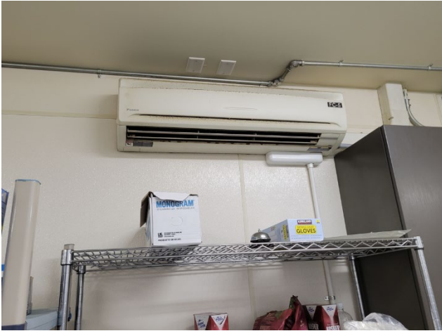
VRF In Kitchen
