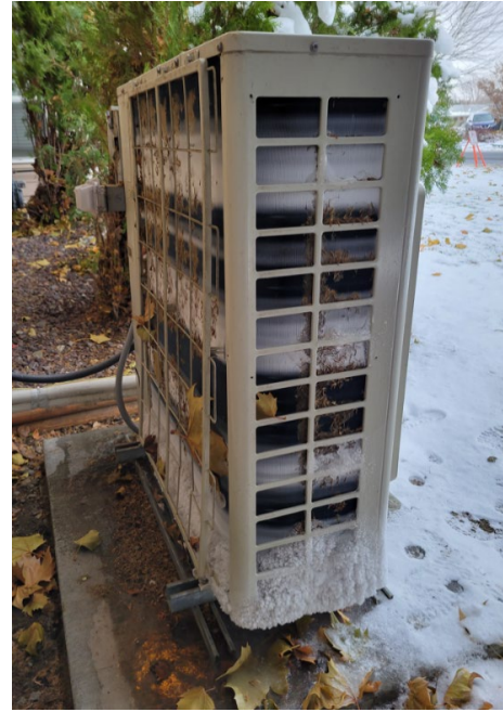
Classroom VRF Outdoor Unit
