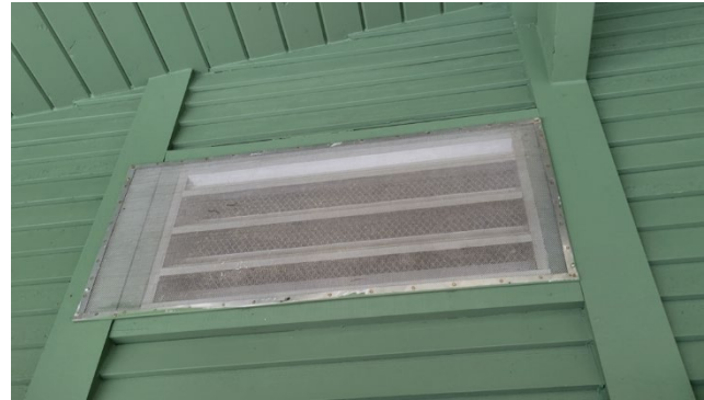
Kitchen Makeup Air Intake
