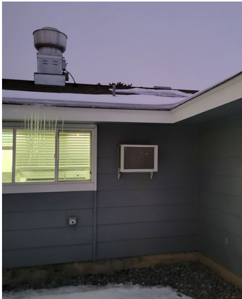
Exterior of Kitchen with Thru-wall AC and Fan.
