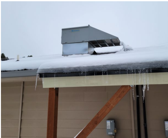
Rooftop Makeup Air Unit
