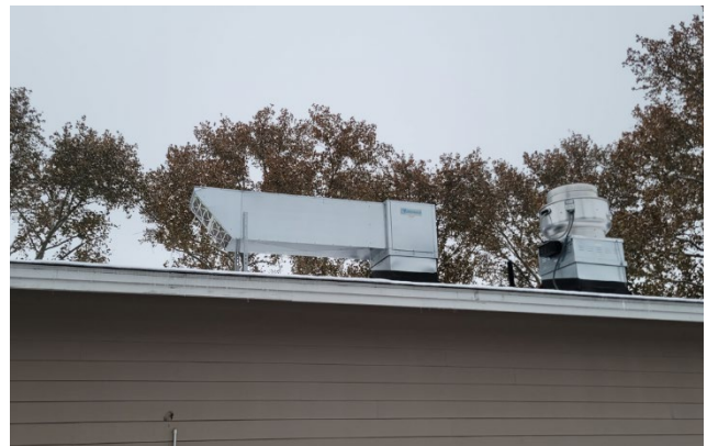
Kitchen Exhaust and Makeup Air
