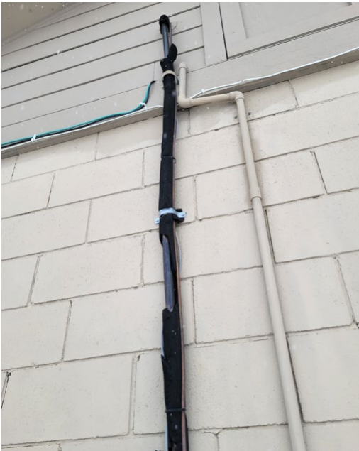
Classroom Refrigerant Piping with Degraded Insulation
