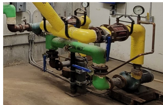
Building (Tertiary) Hot Water Pumps are disabled (Note Valve Position)
