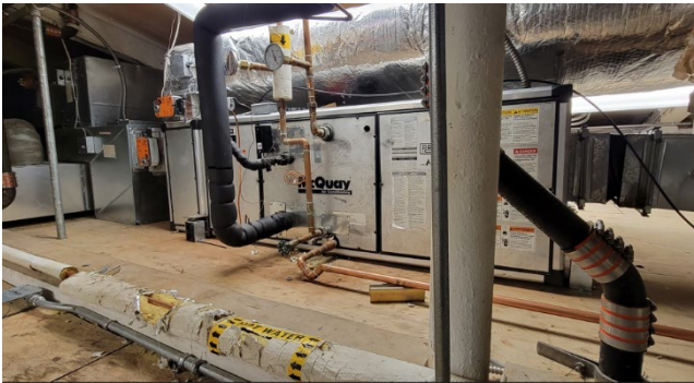
Air Handling Unit
