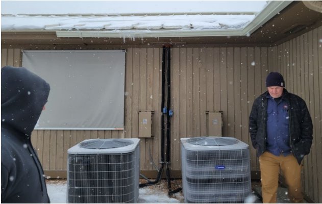
Outdoor Condensing Units for Main Building Furnaces. Refrigerant insulation is unjacketed and degraded
