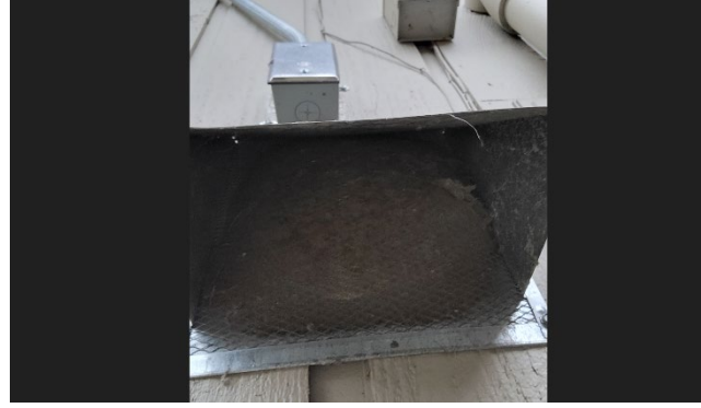
Exterior of Water Heater Combustion Opening Opening is completely clogged with dust and dirt.
