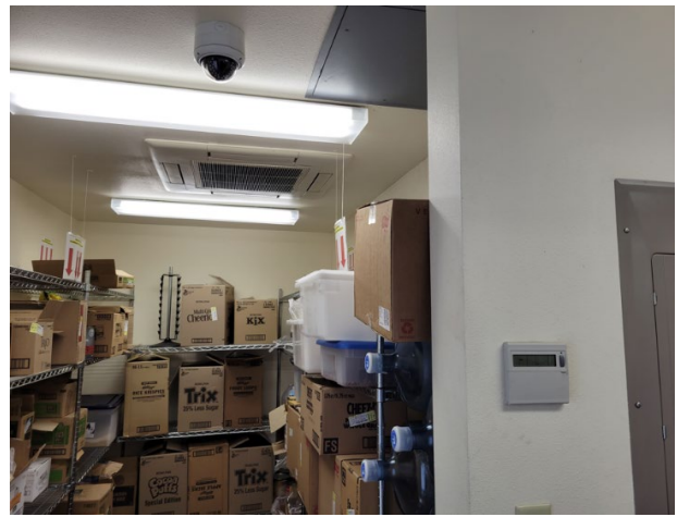
Older AC Unit in Dry Storage Pantry Area
