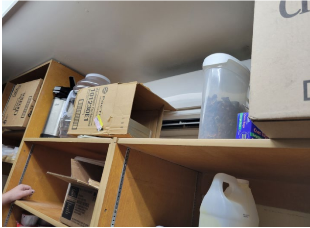
Pantry AC Unit Hidden Behind Stored Items
