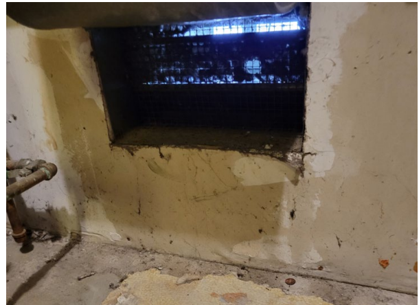
Interior of Water Heater Air Intake Clogged with debris and lint
