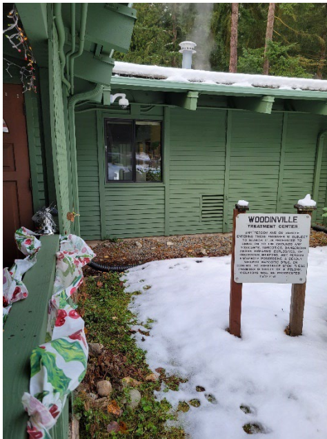
Water Heater Air Intake
