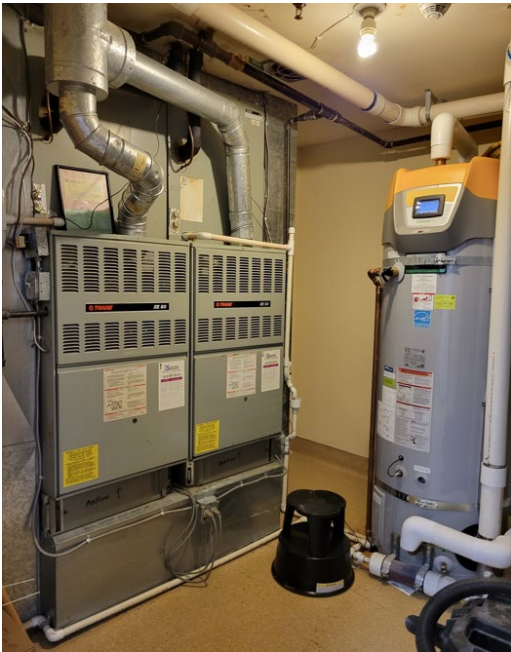
Furnaces (1 & 2) and Water Heater in Electrical Room
