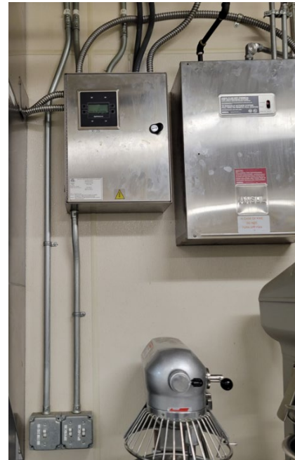
Kitchen Hood and Makeup Air Controller Note: Switches in lower left bypassing controller.
