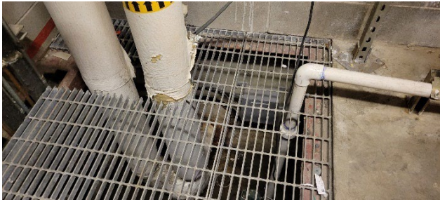
Building S heating water service
