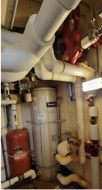
Hot Water Pump Blocked by Domestic Hot Water Pipes
