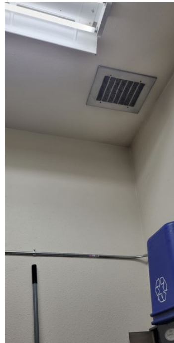
Exhaust fan at janitor nook not working
