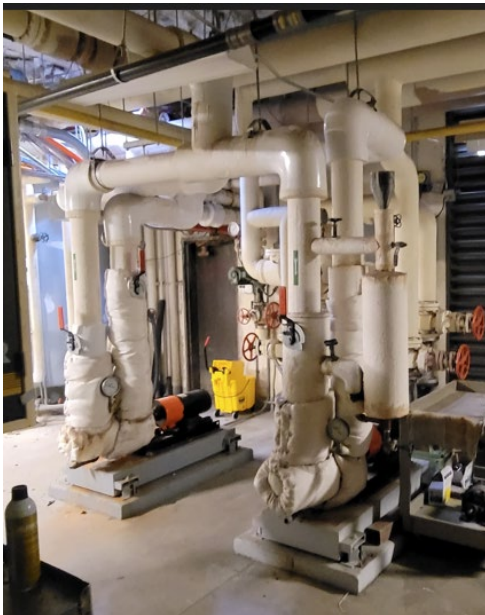
Commissary HHW Pumps
