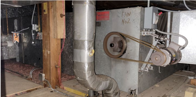
Air Handler Note: One Belt is worn and slipping
