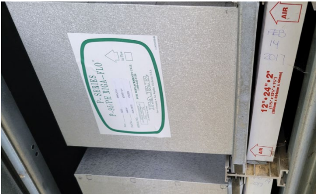
Filters on Recirculated Dust Airflow
