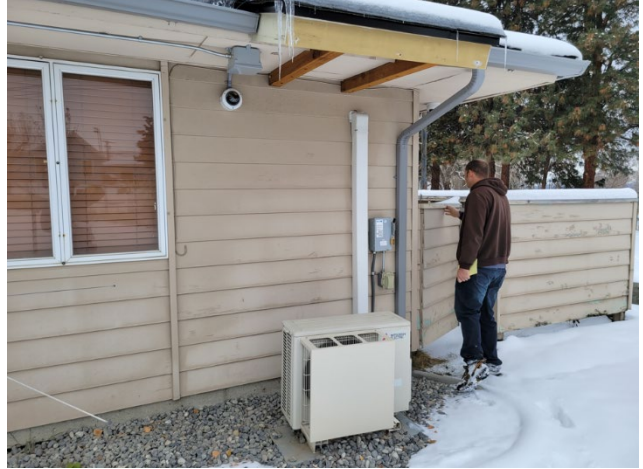
Server Room Outdoor Unit.
