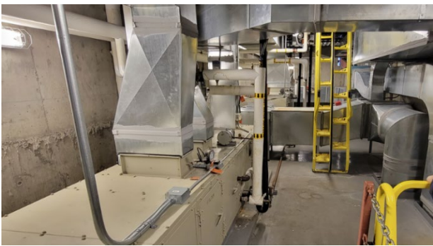
Mechanical Mezzanine with AHUs
