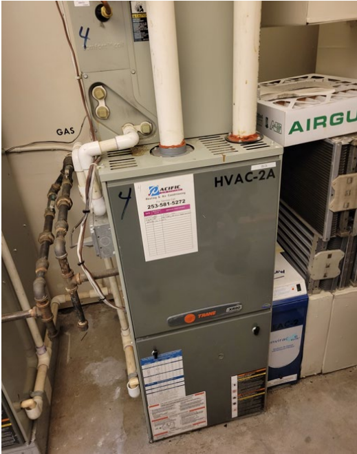
AHU Serving Recreation Room
