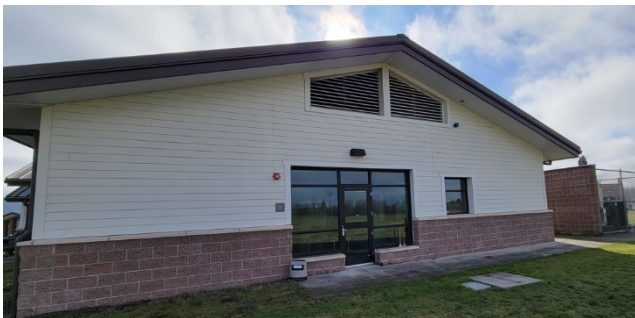
Outdoor Air Intake
