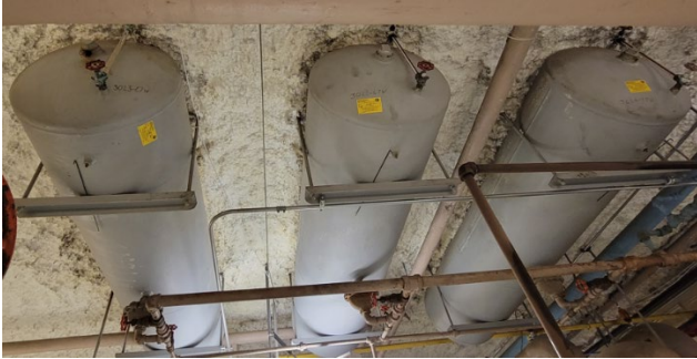
Expansion Tanks Against Ceiling
