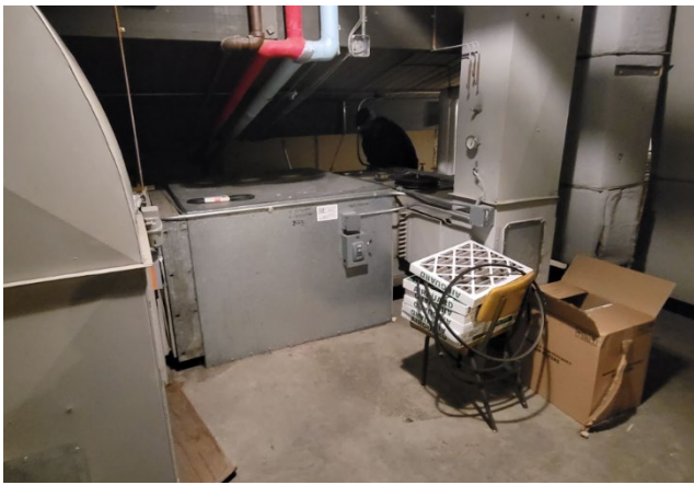
Heat and Vent Unit Serving Locker Rooms
