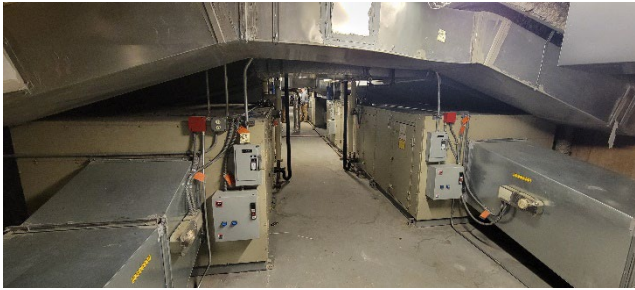
Mechanical Mezzanine and Air Handling Units
