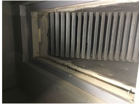
Typical Return Intake
