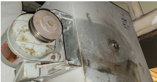
Unit for Weight Room and Offices with Broken Fan Shaft
