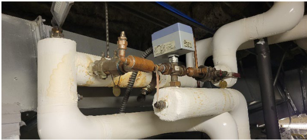
Typical AHU 3-way control valve.
