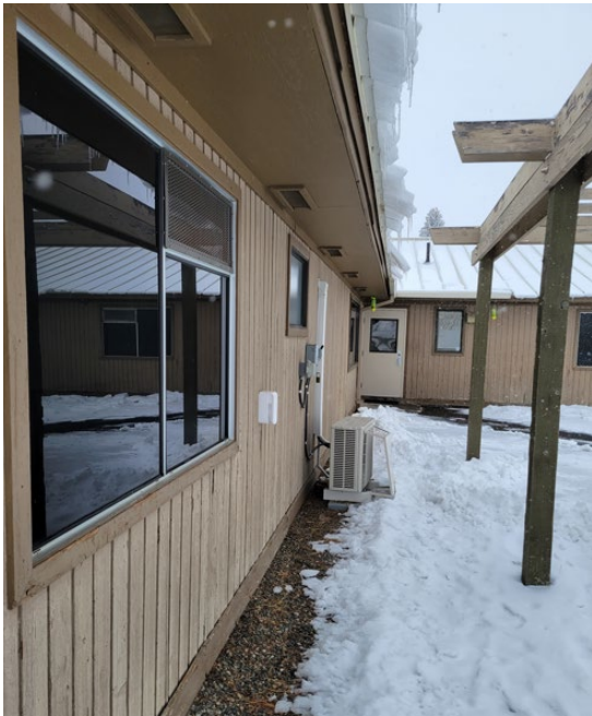
Server Outdoor Unit Located Directly Below Roof Edge
