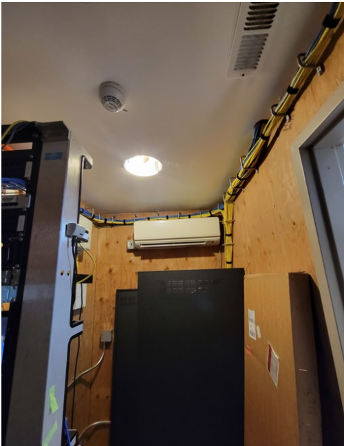
Server Room AC Unit Indoor Section
