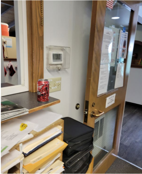
Thermostat in Reception Office Controlling the Basement Furnace
