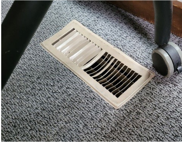
Floor Register in Living Room
