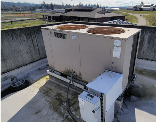
Condenser unit for AHU-F2
