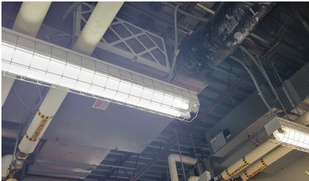
Fan Powered Terminal Units
