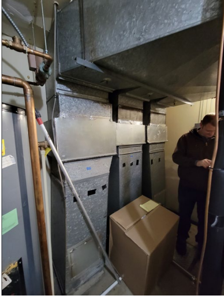
Duct branches appeared to previously have reheat coils controlling temperature separately to different areas.
