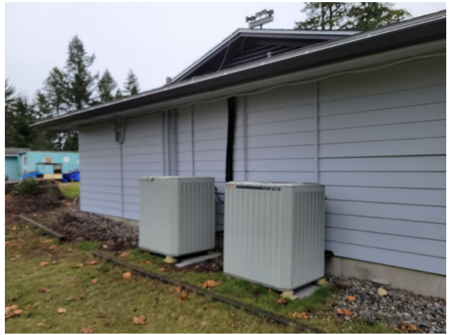
Condenser Units Serving Furnace 1 & 2
