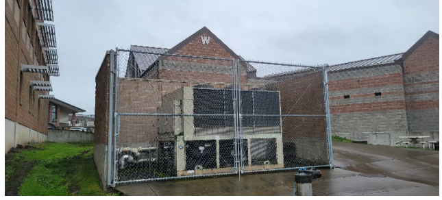
Chiller Serving HCA and IMU
