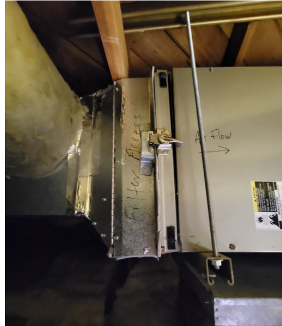
Office Unit Filter Section
