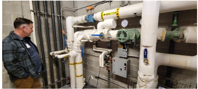
Building S interior heating water pumping station (Tertiary)
