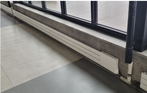
Baseboard Heaters at Dining Curtainwall
