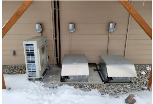
Pantry Outdoor Unit and Refrigeration
