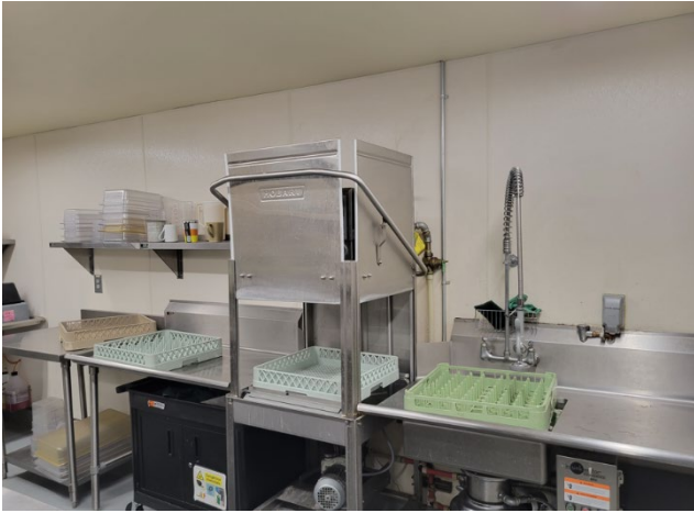
Kitchen Dish Area No Exhaust
