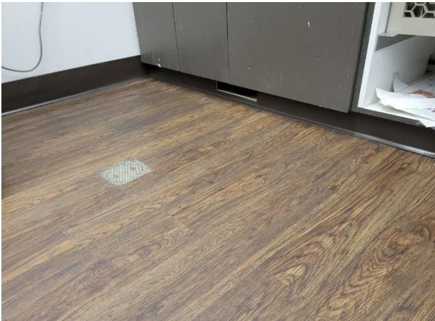
Toe Kick Outlet to Unit #1 with no Grille 120 CFM
