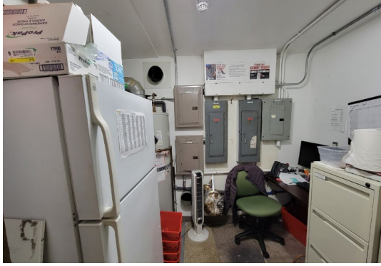
Utility Area with Kitchen Office, Water Heater, and Electrical Gear.
