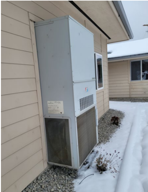
Classroom Wall Mounted AC Unit
