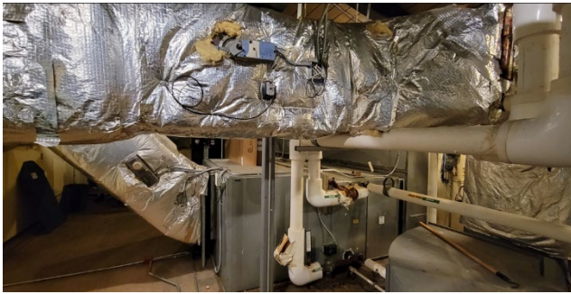
Mechanical Mezzanine Dining AHU, abandoned legacy damper actuator for variable flow operation
