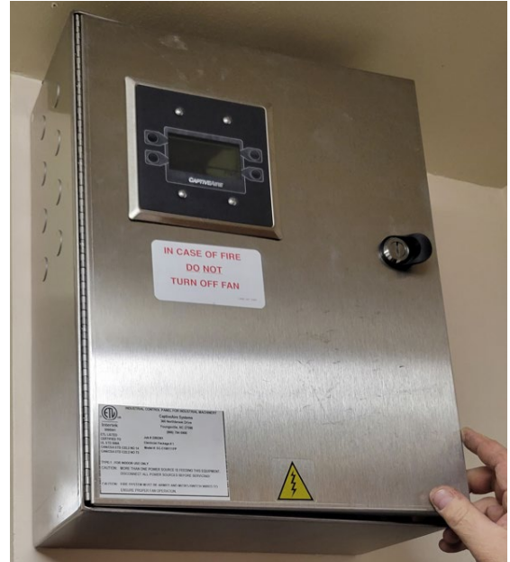
Exhaust and Makeup Air Control Box. Note display is damage and unusable
