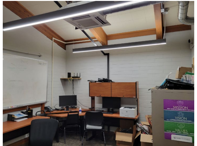
Office on VRF System and Unit #1
