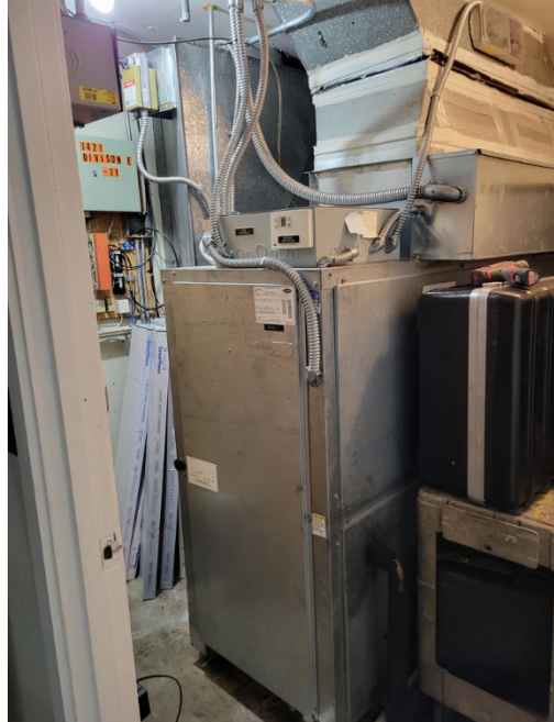
Mechanical Room with AHU-1
