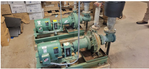
Heating Water Pumps
