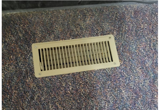
Typical Floor Register
