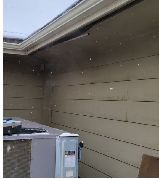
Flue Gases Rising to roof edge appear to be damaging structure
