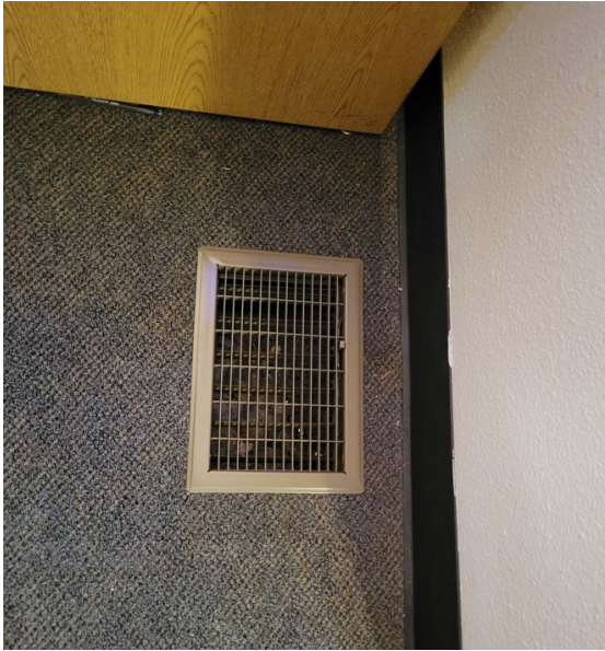
Typical Floor Grille
