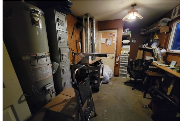
Workshop with Classroom Building Furnace
