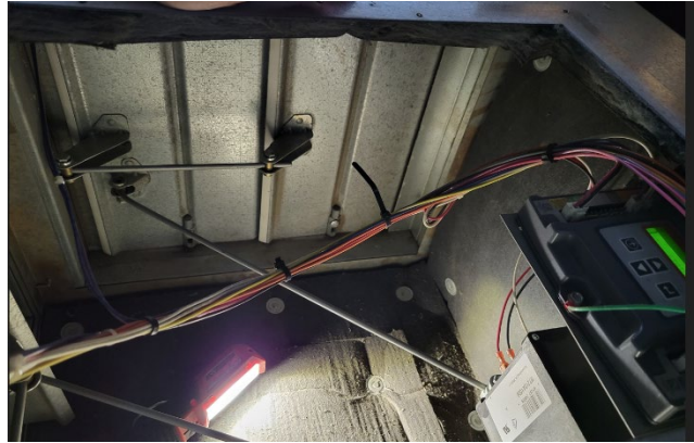
Outdoor Air Damper and Broken Actuator
