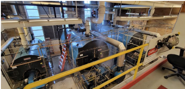
Boilers from above, outside control room
