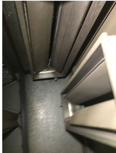
AHU-S1 Mixing box
