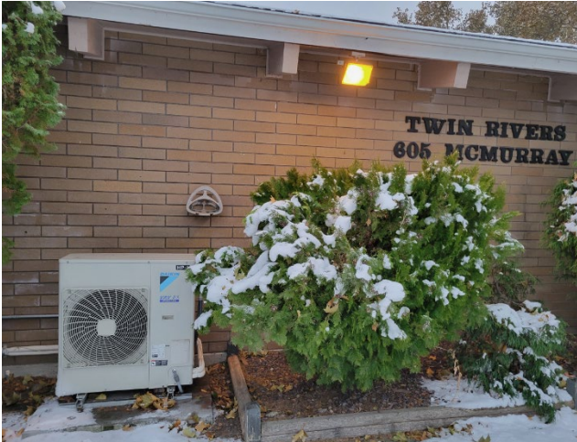
Classroom VRF Outdoor Unit
