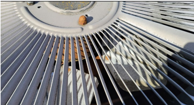
Condenser unit for AHU-F1
