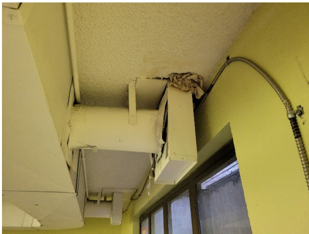
Ductwork to Furnace System Floor Grille
