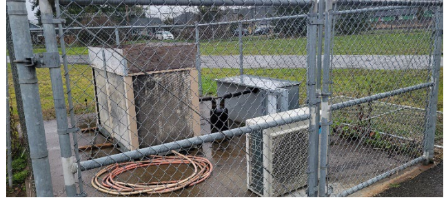
Outdoor Condenser Equipment for AHU-A1 and Server AC Not: Improvised addition of extension to reduce recirculation of hot discharge air and sprinkler to reduce ambient temperature
