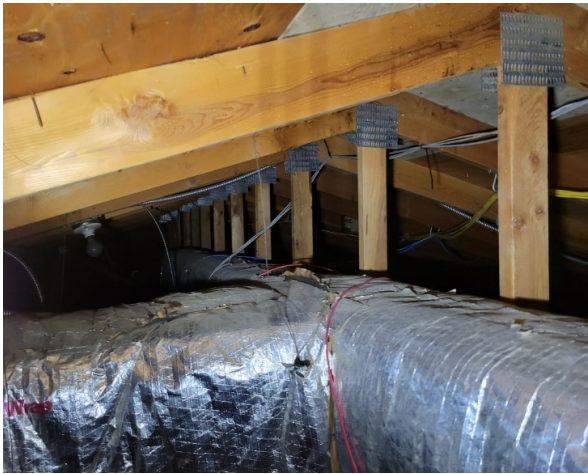
Attic Return Duct
