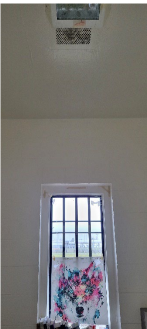
Sleeping room, ceiling return grille
