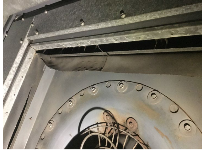
AHU-S4 Supply Fan With torn flexible connection
