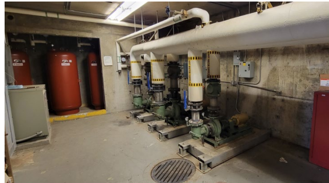
Primary pumps and expansion tanks at lower level
