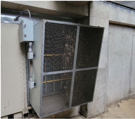
Air Intake in Area Well with Airflow Station
