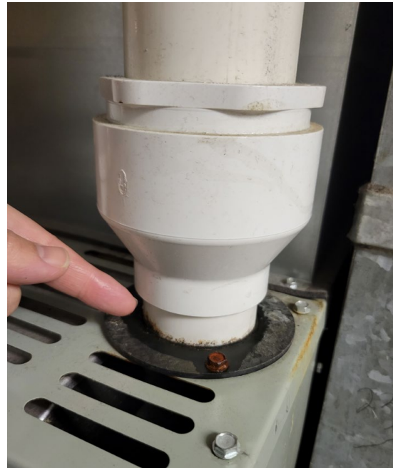
Flue Connection Leaking
