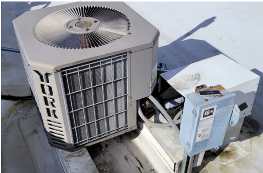
Condenser unit for AHU-F1
