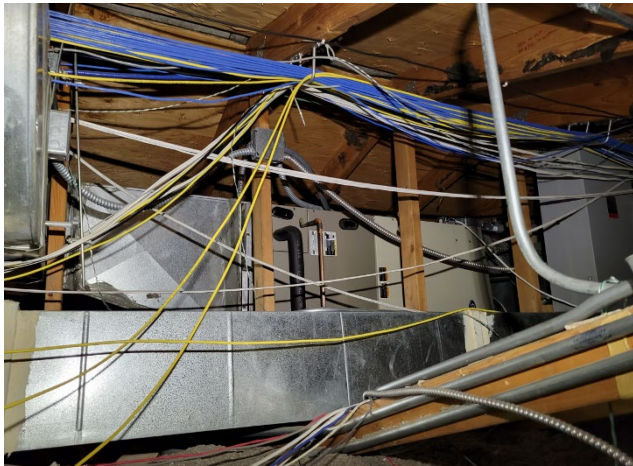
East Side AHU
