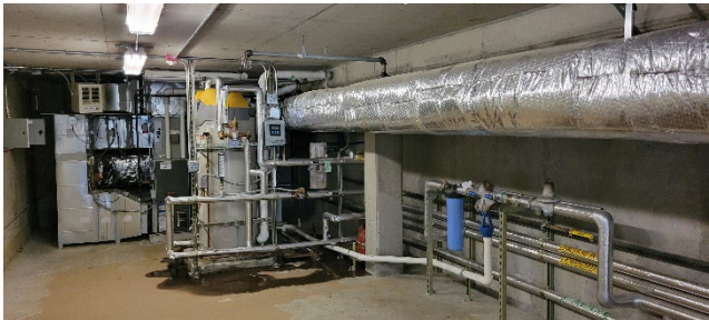
Mechanical Room with Water Heater and Furnaces
