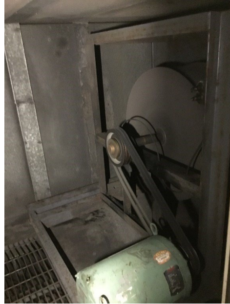
Supply Fan Supply to building via grate in lower left
