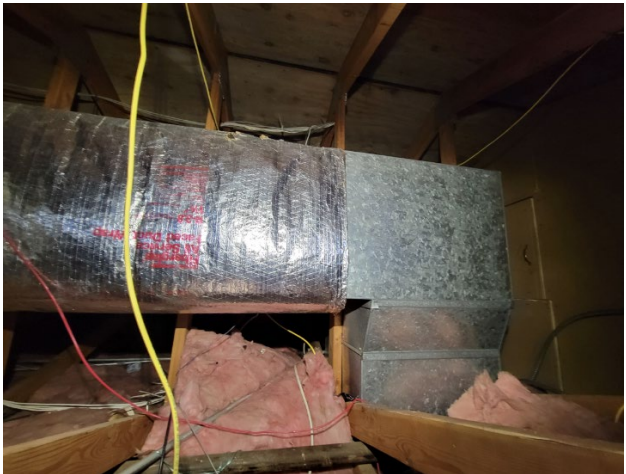
Attic Return Duct
