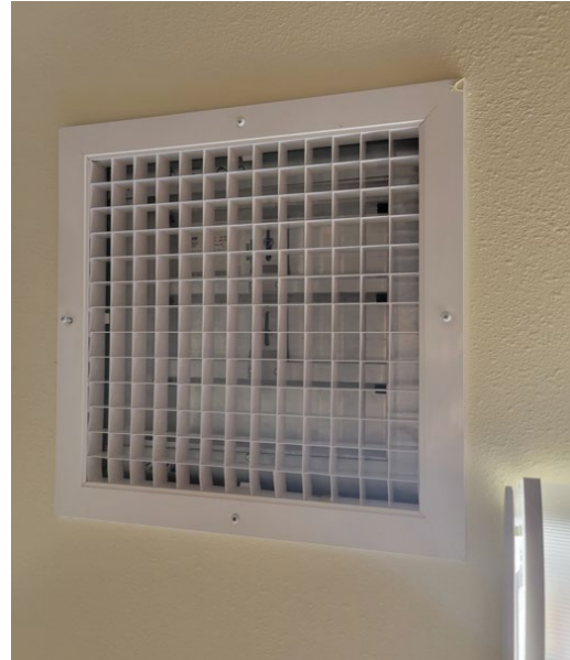
Transfer Grille Between Kitchen and Dining. Note this is not working because it includes a barometric damper that is not adjusted properly (no weight).
