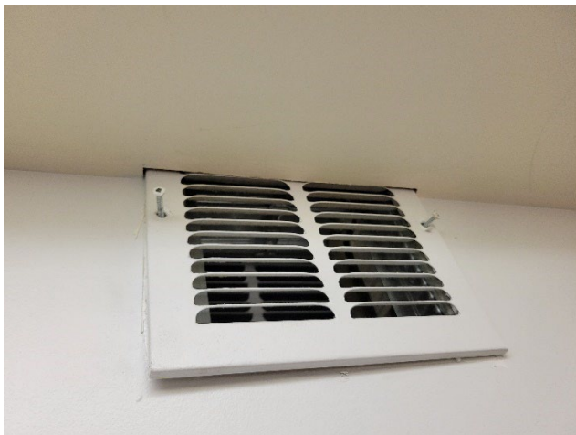
Typical Bedroom Transfer Grille from Hall Partially blocked by furring installed around fire sprinkler pipe
