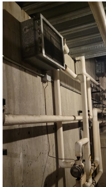
Typical supply branch to below-grade duct with heating coil. Pneumatic Control Valve that originally responded to thermostat is disabled.
