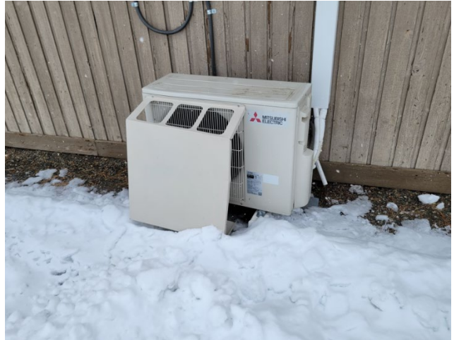
Server Room Outdoor Unit Note: Damage from Snowfall
