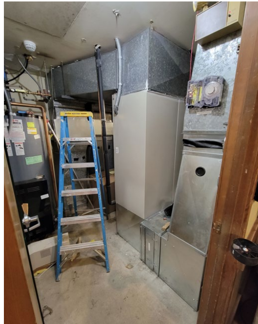
Mech Room with Furnace
