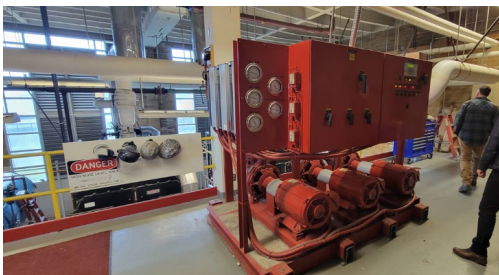
Upper Level with secondary pumps overlooking boilers
