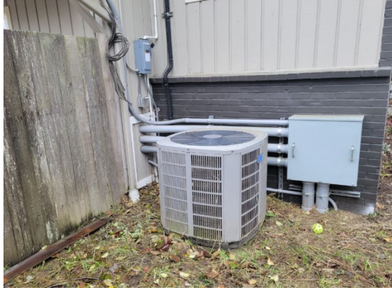
Condenser Unit Serving Upper Floor
