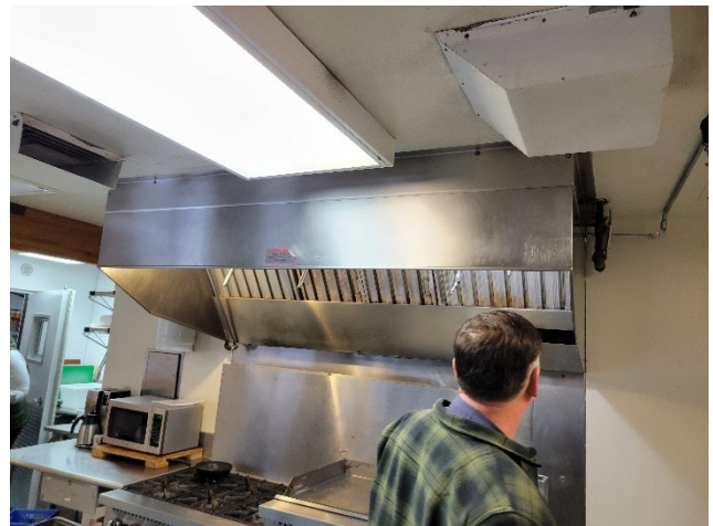
Kitchen Hood and Makeup Air Diffusers with Fabricated Shields
