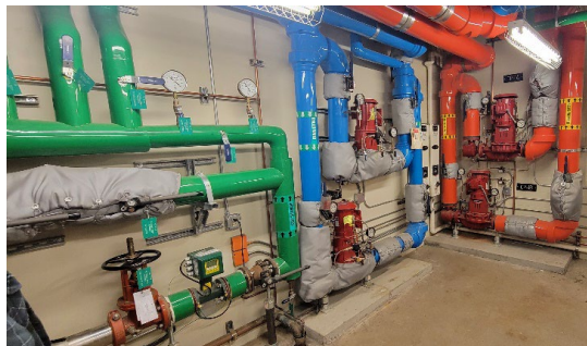
Building C Pumps
