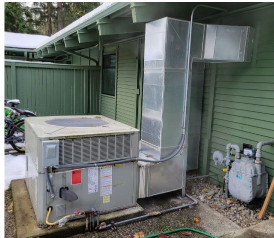
Gas Fired Packaged AC Unit Serving Bedrooms No Outdoor Intake. Note gas pipe is rusting where combustion flue discharges directly onto it
