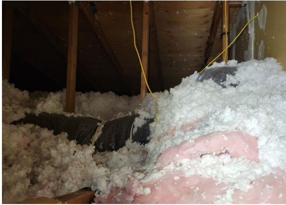
Attic Ductwork Covered with Insulation
