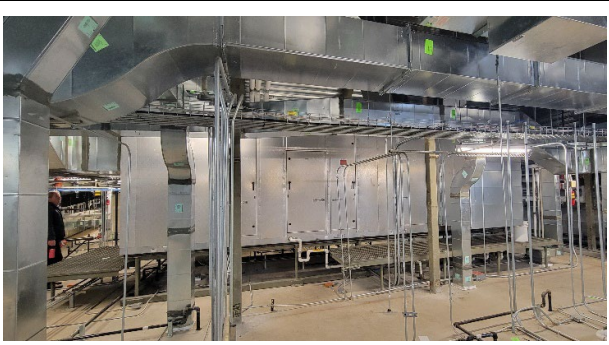
Mechanical Mezzanine and MZU-1
