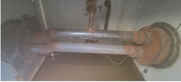
Pipe branch from main.
