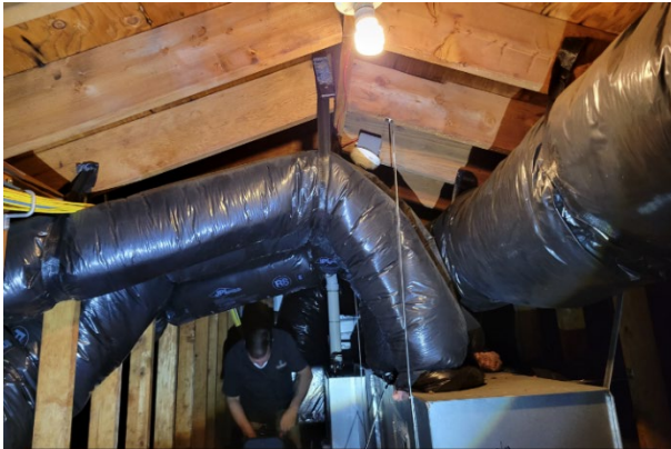
Second Floor System Supply Ductwork in Attic
