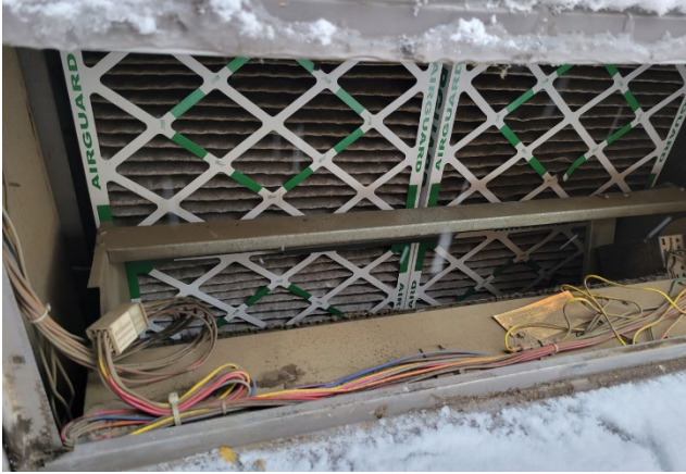
Interior of Unit, Filters
