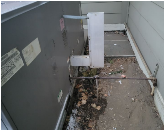
Condensed Flue Gases Freezing onto Gas Piping
