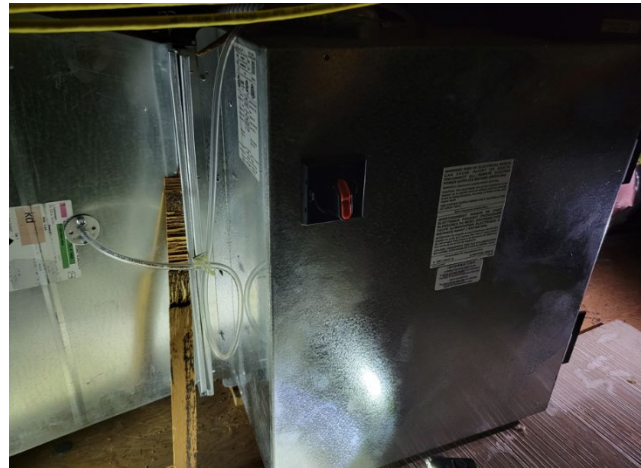
Kitchen Makeup Electric Heater
