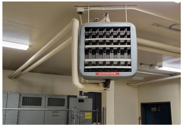
Loading/Receiving Area Unit Heater
