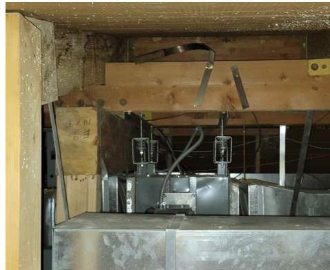
Exhaust Fans in Attic
