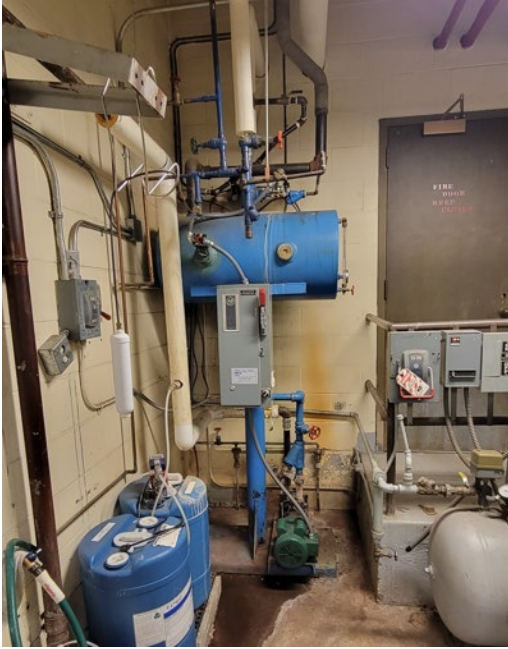
Steam System Feedwater Pump Assembly
