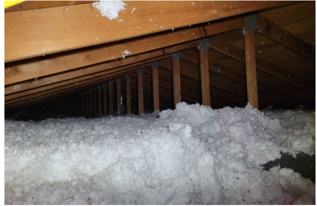
Attic Ductwork Covered with Insulation
