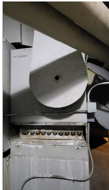
Heat and Vent Unit Serving Gym
