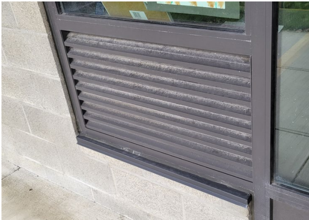
Typical Unit Vent Outdoor Air Intake Integrated Into Storefront Glazing
