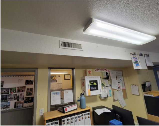
Typical Sidewall Register in Soffit
