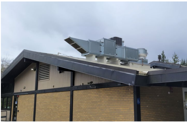
Rooftop Kitchen Exhaust and Makeup Air Unit
