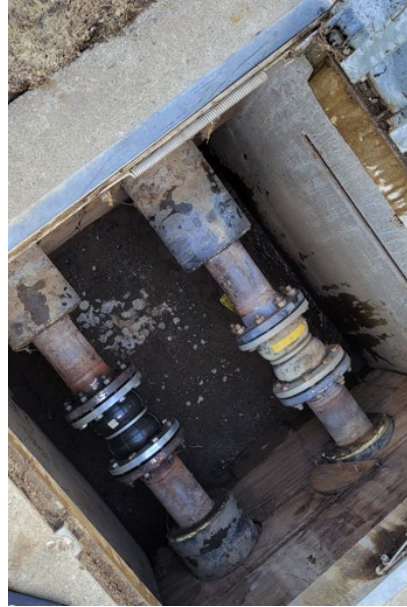
Small vault for expansion couplings on branch piping. Coupling on the left replaced after bursting.
