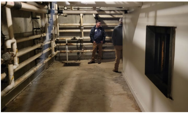
Basement Supply Air Plenum with zone heating pipe and sump pit. View of central corner from West
