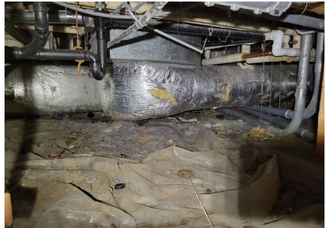
Ducts Entering Building Crawlspace
