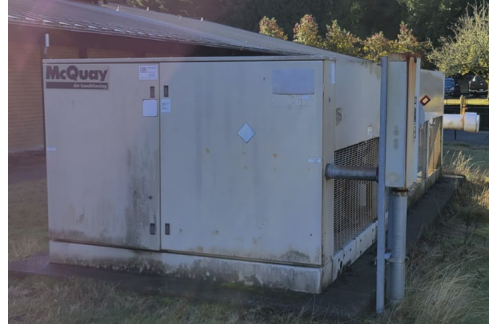
Campus Air Cooled Chiller
