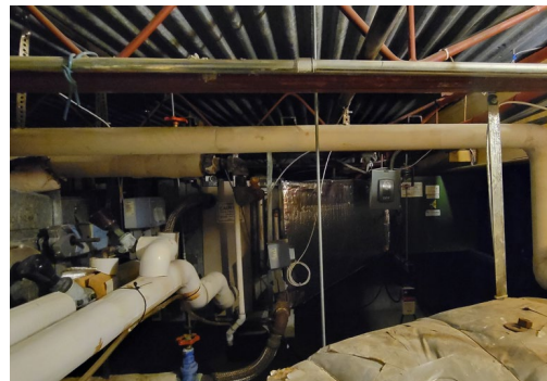
Social Services AHU
