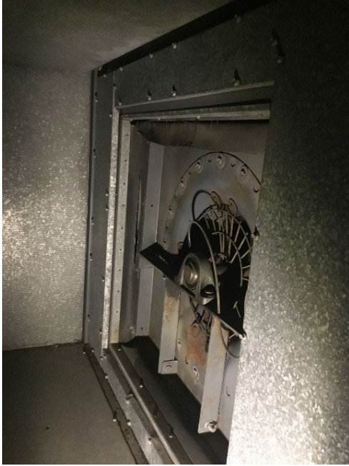
AHU-S4 Supply Fan Note: Torn flexible connection
