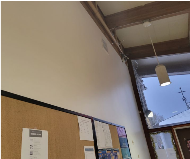
Classroom ERV Relief Air Discharge in Entryway
