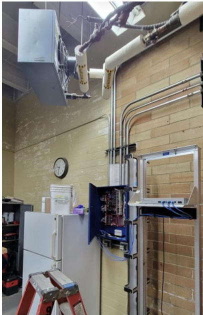
Unit heater and central plant controller in upper-level workshop
