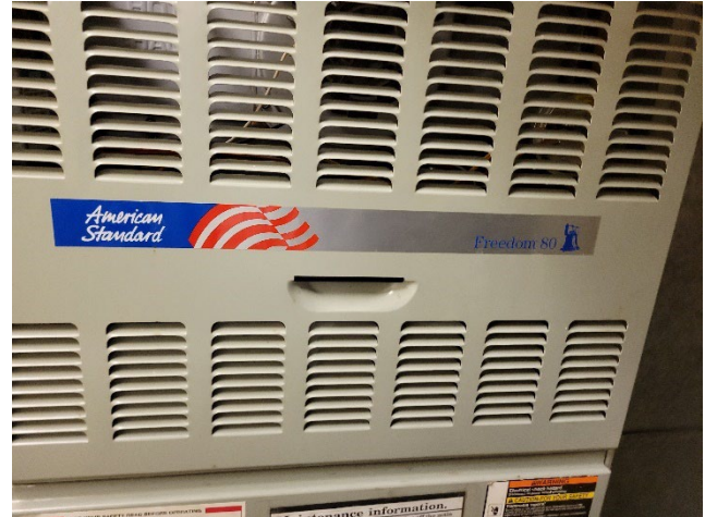
Furnace Serving Common Space and Office
