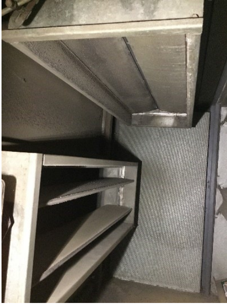
AHU-S2 Mixing Box Note: Outdoor air damper is closed.
