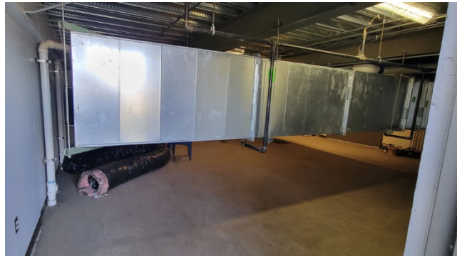
Maintenance Access to HCA Equipment is Below this Duct
