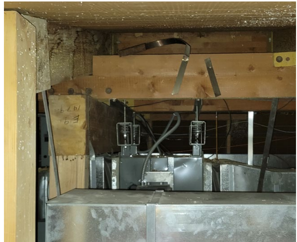
Exhaust Fans in Attic
