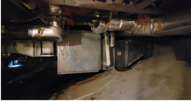
Health Center AHU AHU and intake ductwork are partially set into the retaining wall
