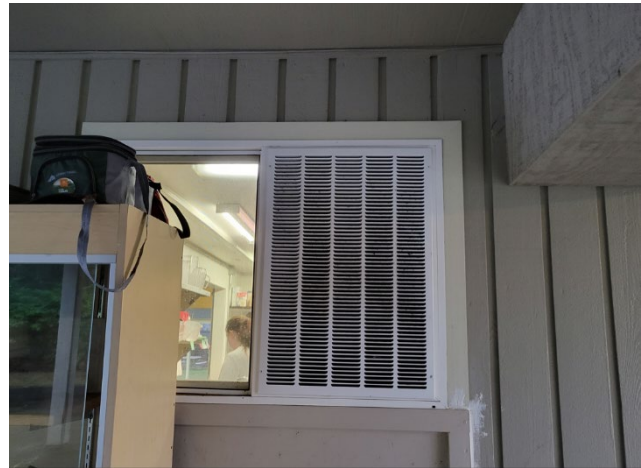
Exterior of kitchen intake is a residential interior grille
