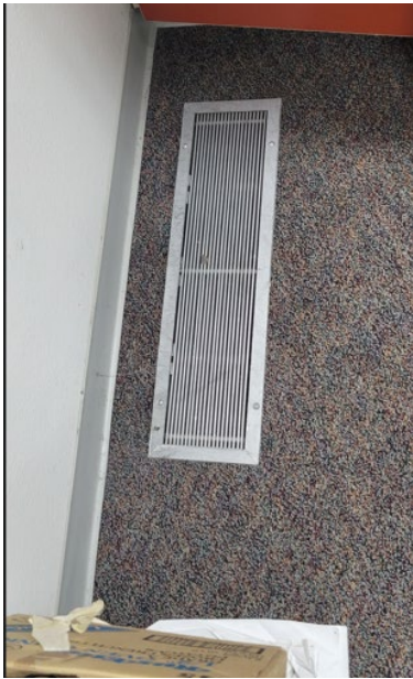
Typical Floor Grille
