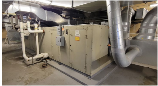
Building D Mechanical Mezzanine
