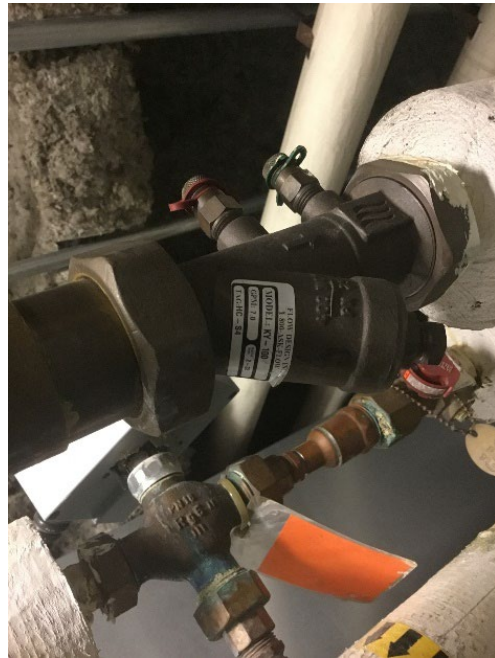
Automatic flow control valve
