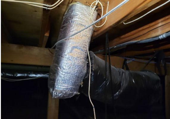
Typical Connection to Floor Grille
