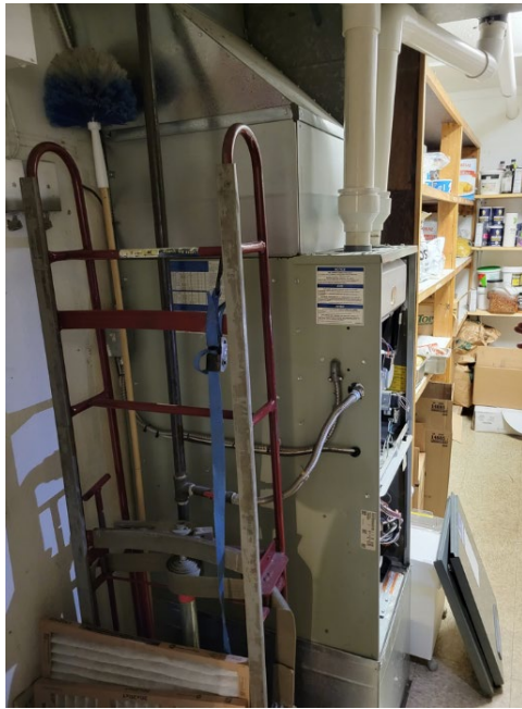
First Floor Furnace
