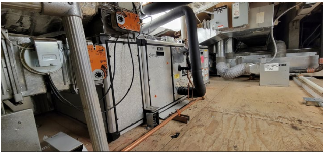
Attic with AHUs and Exhaust Fans
