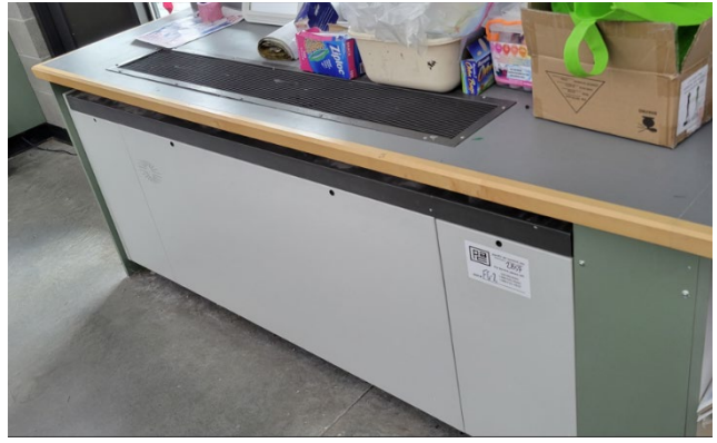
Unit Ventilator in Art Room
