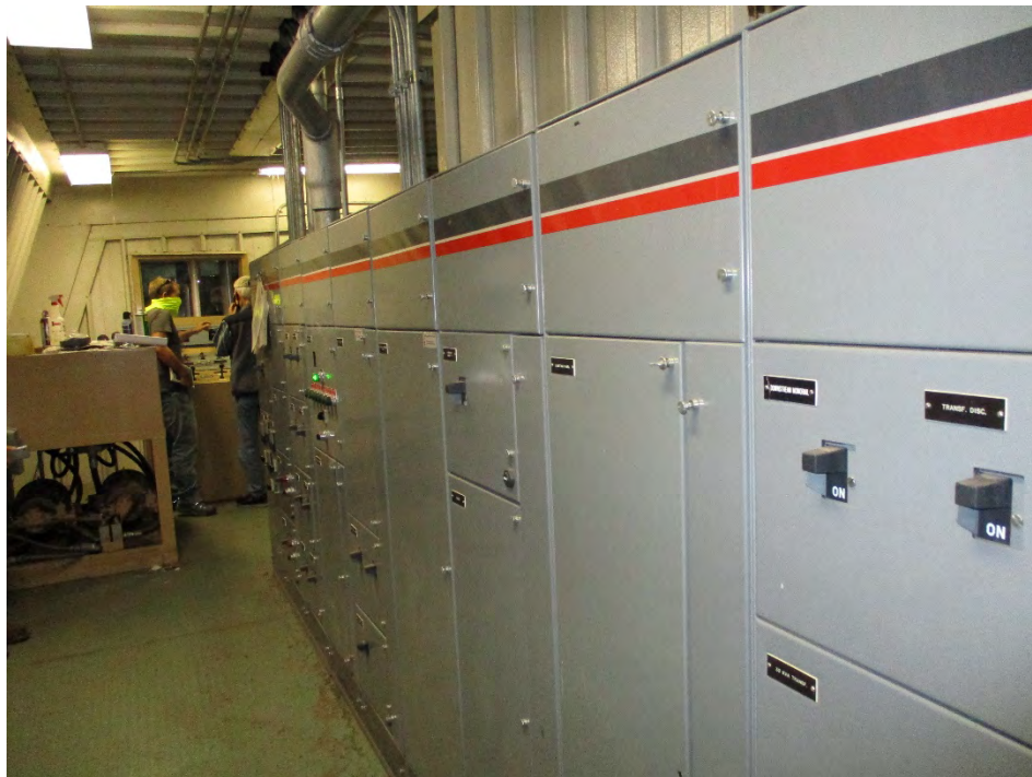
Figure 17 – MCC Line Up
