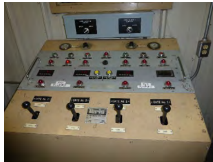
Figure 23 – Existing Control Console
