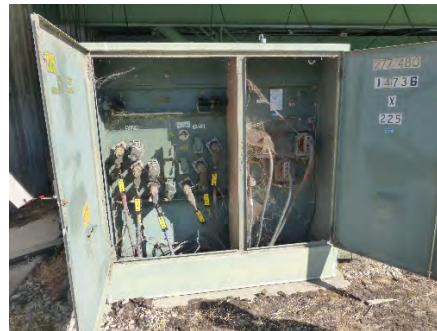
Figure 33 – Existing Pad-Mount Transformer with Doors Open
