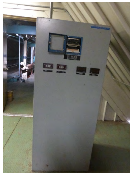
Figure 35 – Abandoned Control Panel
