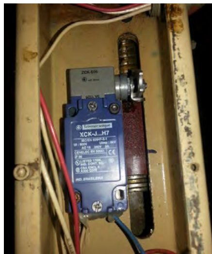
Figure 28 – Gate Travel Limit Switch
