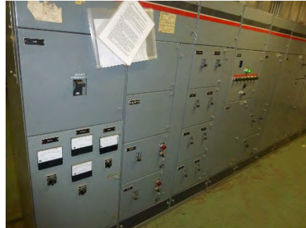
Figure 24 – Existing MCC Lineup
