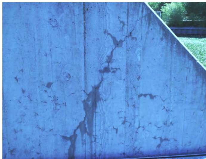
Figure 3 – Showing Crack in East Wall Downstream End
