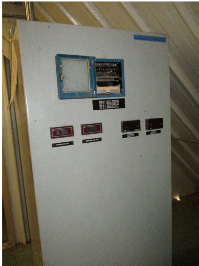
Figure 15 – Project Monitoring Panel (Non-functional)
