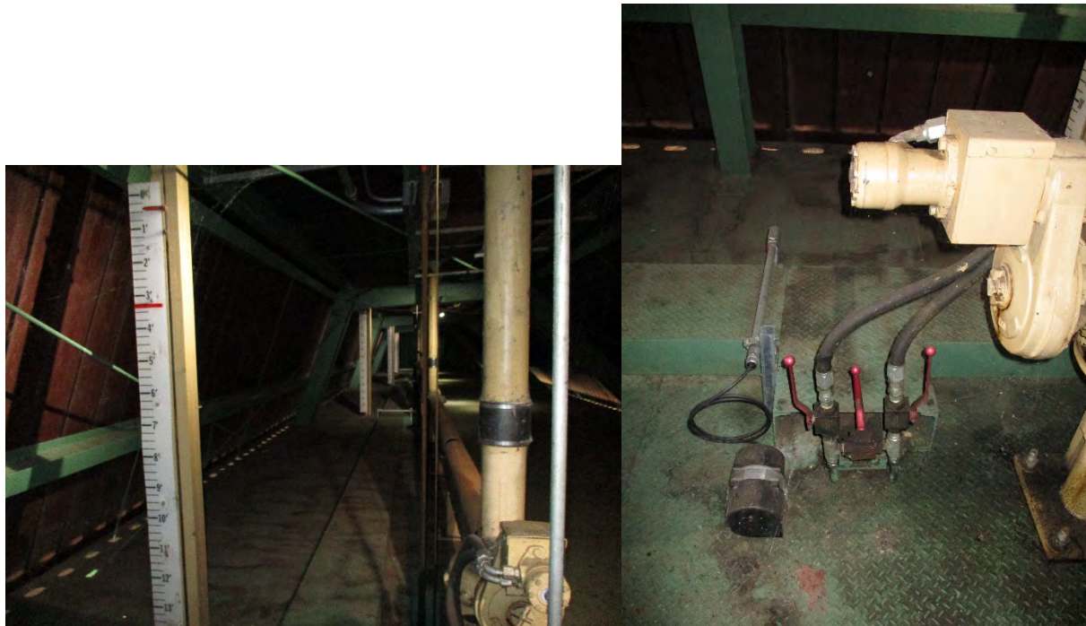
Figure 6 – Spillway Gate Lifting Equipment
