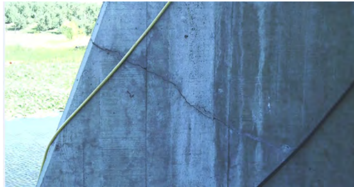
Figure 2 – Showing Crack in East Wall Upstream End
