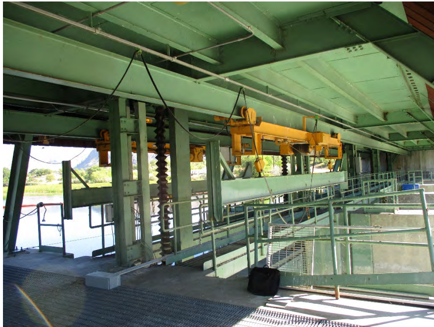
Figure 16 – Stop Log Handling Equipment
