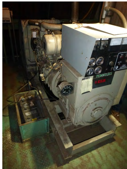
Figure 25 – Existing 50-kW Backup Generator
