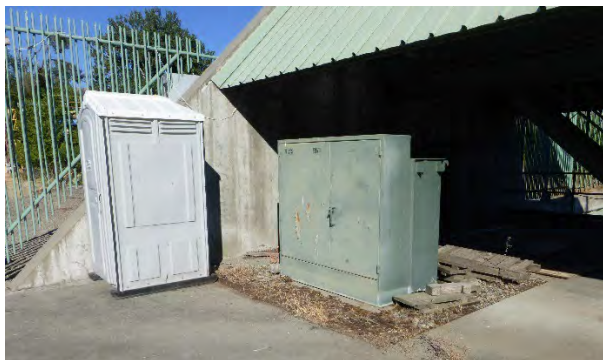
Figure 22 – Main Transformer Owned by Okanogan PUD
