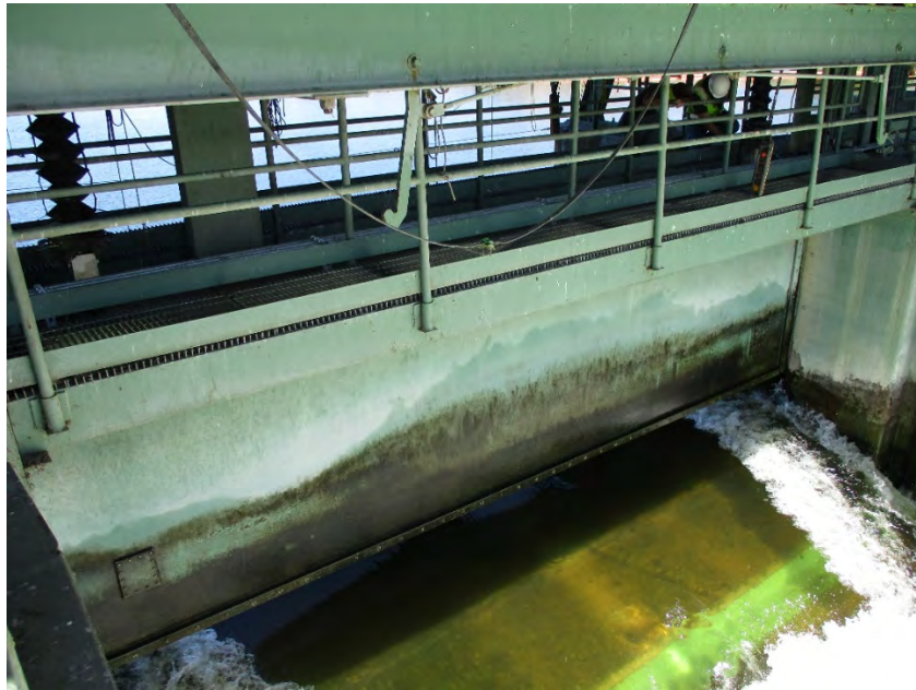
Figure 10 – Gate #1 Fully Open (from downstream)
