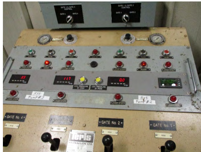
Figure 8 – Hydraulic Control Panel
