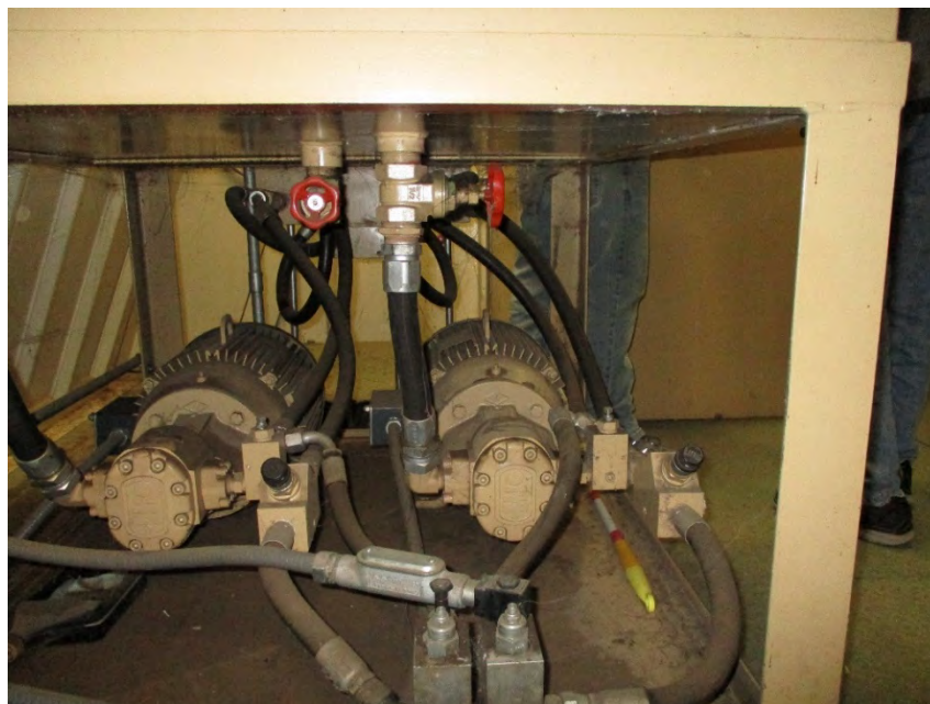
Figure 7 – Hydraulic Power Unit
